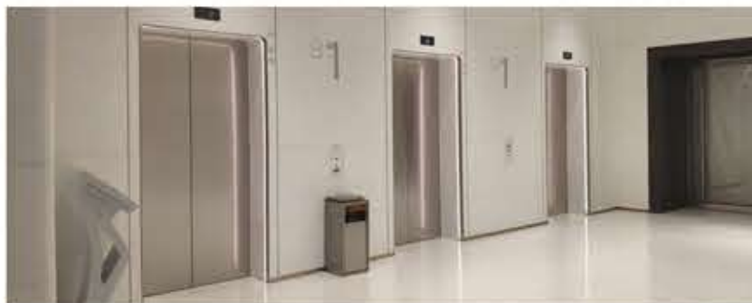
Automatic Lift Facility
